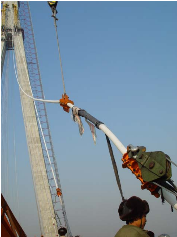
Erecting the 228 meters long cable no.10 on the Sutong Bridge over the Yangtze River.
