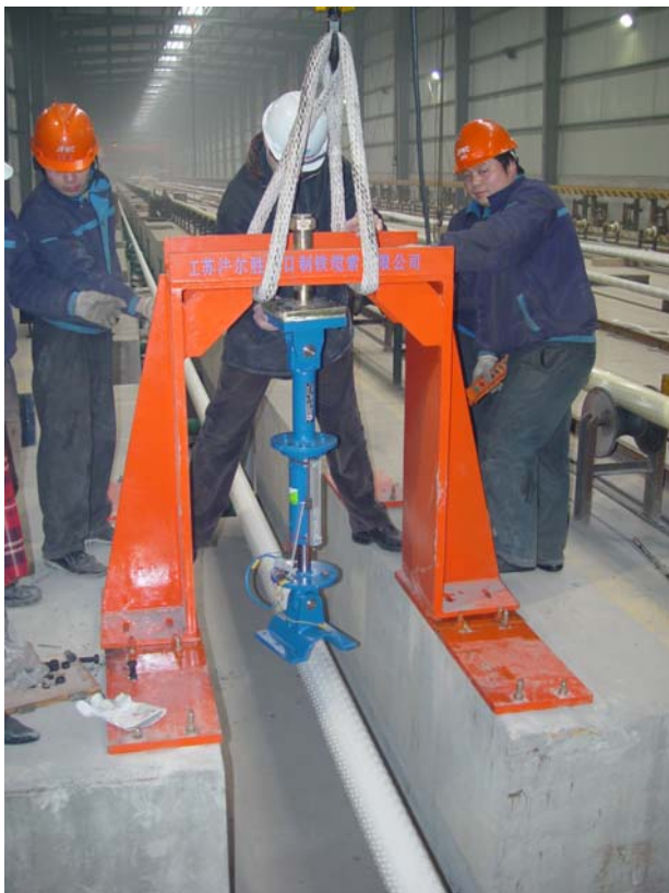
Mounting the MR damper to the test cable at 6.6 meters from the anchor.
