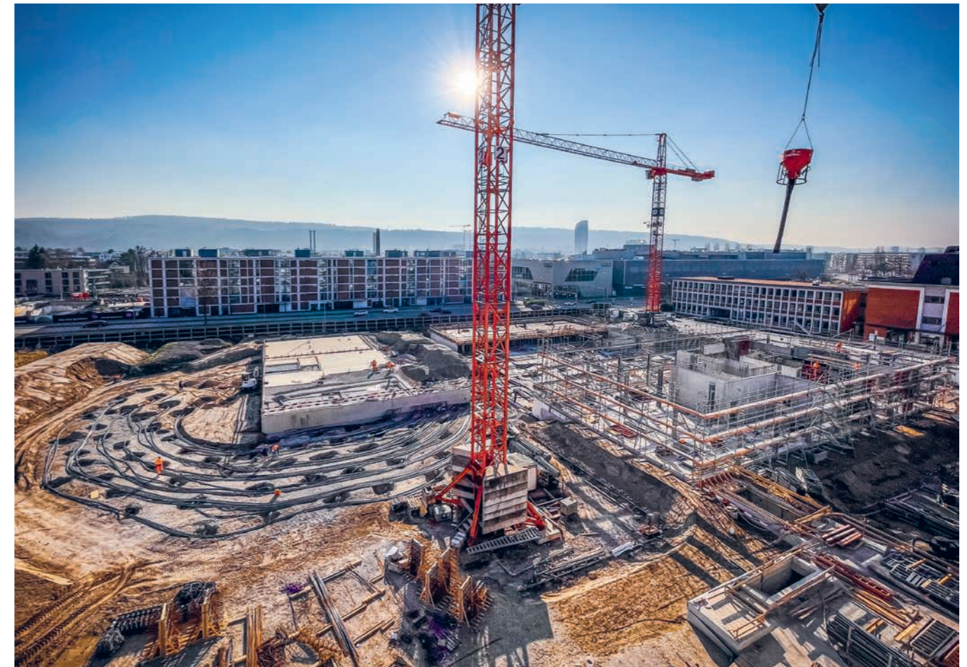
View of the construction site of the co-operate campus extension, under whose building a geothermal borehole field with 144 geothermal probes reaching down to a depth of 100 meters is being built (left in the picture).
