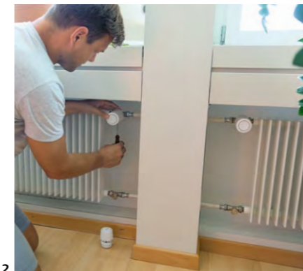
2 The conversion from analogue to smart thermostats connected to the viboo cloud solution is easy to implement in existing buildings and achieves energy savings of between 20 and 40 percent.
