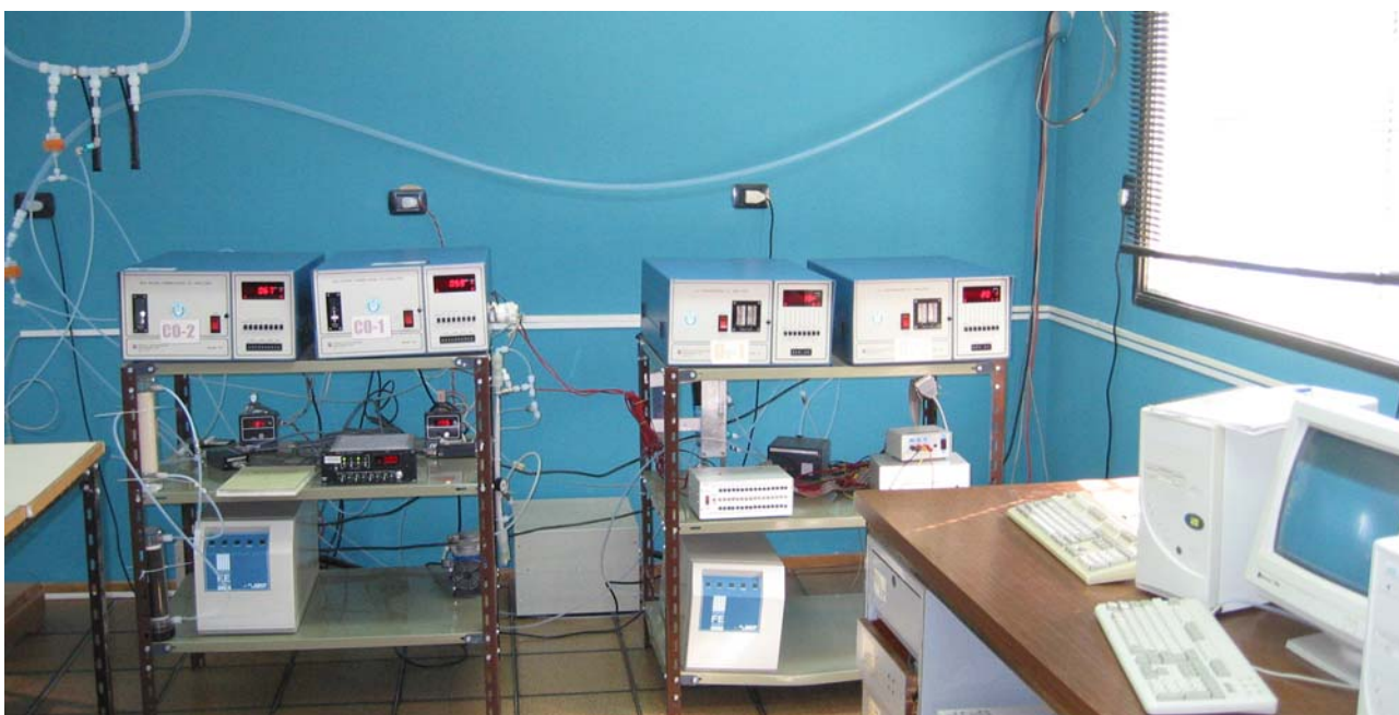
Figure 7: Ozone and carbon monoxide instruments at the Ushuaia GAW station
