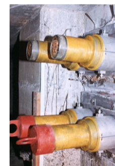
Anchorage of the four CFRP-cables where the forces and the pull-in of the CFRP-wires are measured
