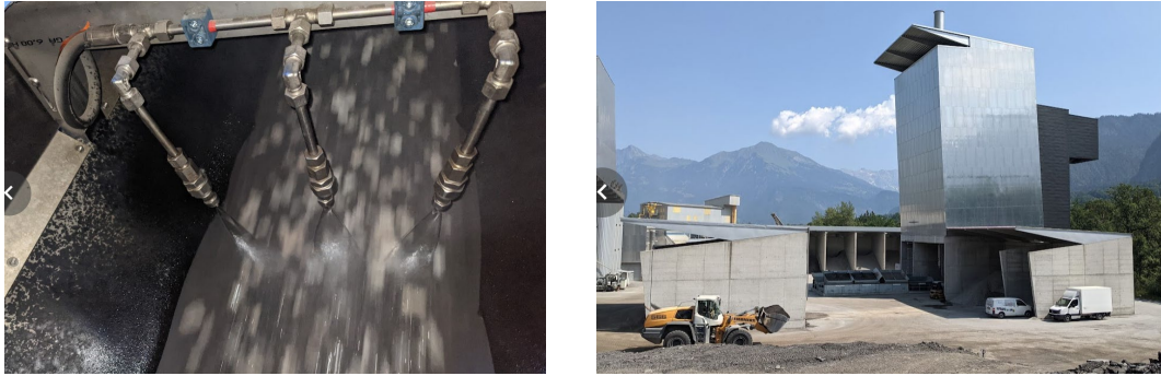
Fig. 149 Rejuvenator addition nozzles over cold material feed belt (left) and Catram AG asphalt production plant that was used for the production of AC F 22 type mixtures (right)
